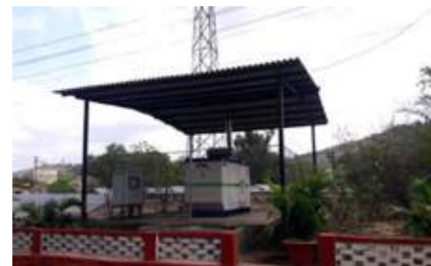
New bigger horse power water pump and 125 kva generator
